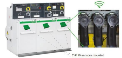
Fig. 1 Example of a Schneider-Electric Ring Main Unit. Detail of GIS shielded termination and external thermal sensors.
