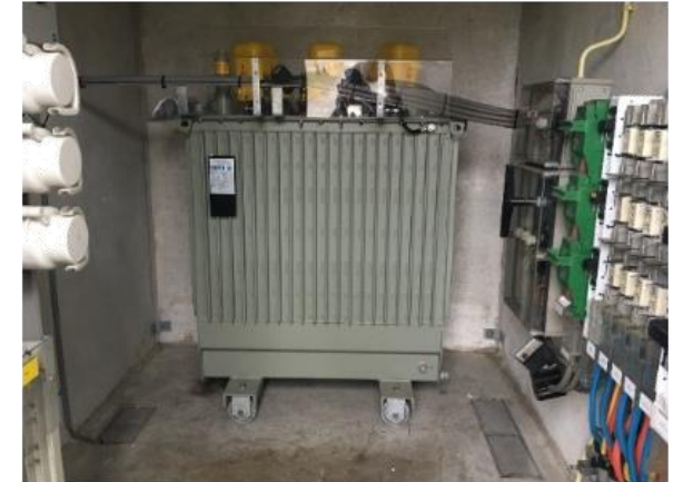
a) Conventional transformer
